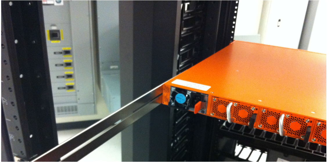
Figure 3-4: Rear View of the Mounted Node and Rails on the Four-Post Rack
