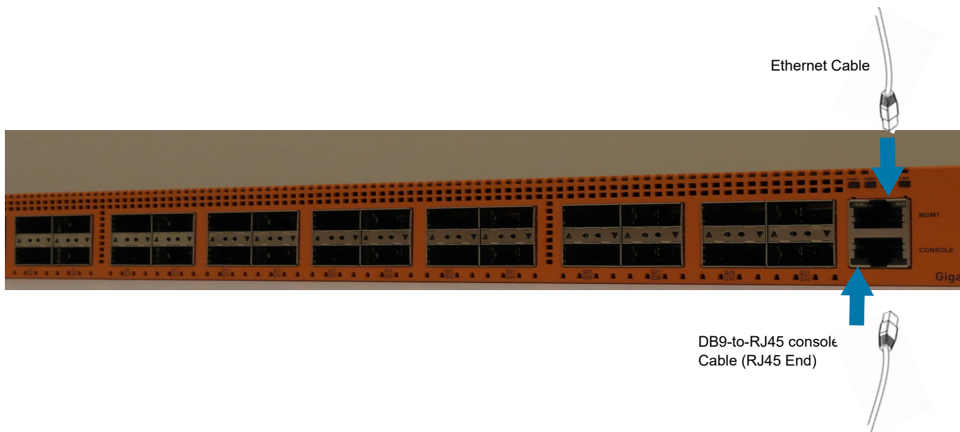
Figure 4-8: Connecting the Console and Management Ports
